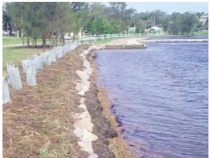
Foreshore stabilisation works involving beach construction and vegetation plantings at Warners Bay
