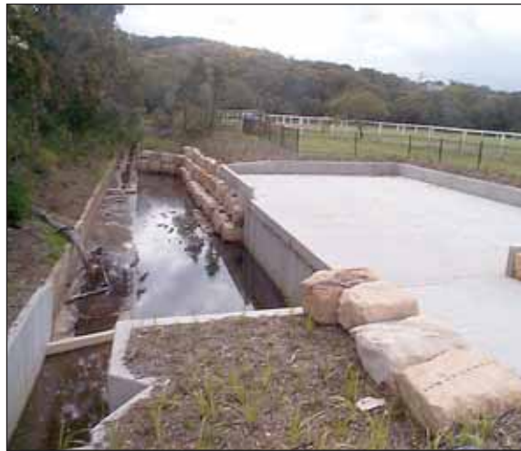
Sediment trap and vegetated basin at Park Avenue, Caves Beach
