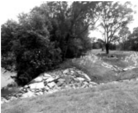
Vegetated drainage swale at Ridley Street, Edgeworth
