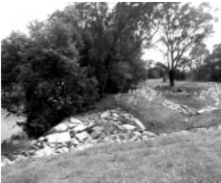
Vegetated drainage swale at Ridley Street, Edgeworth
